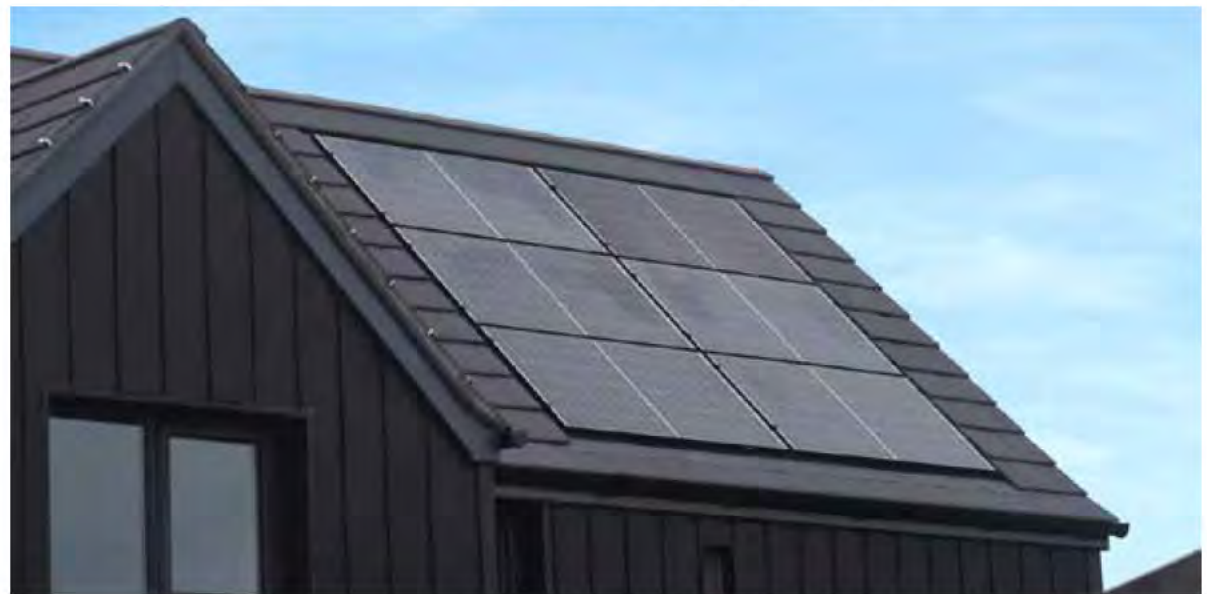
Solar Panel Detailing in Ockford Ridge Development by Thakeham in Godalming
