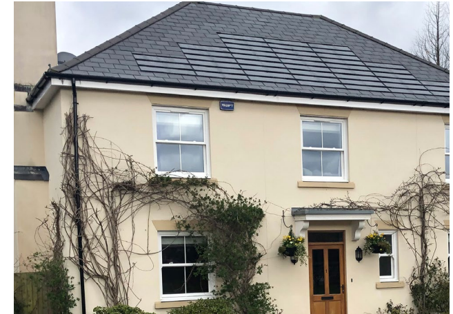
Figure 131: Use of single-like solar panels on a slate roof with the design and colour of the panels matching those of the adjacent slate tiles
