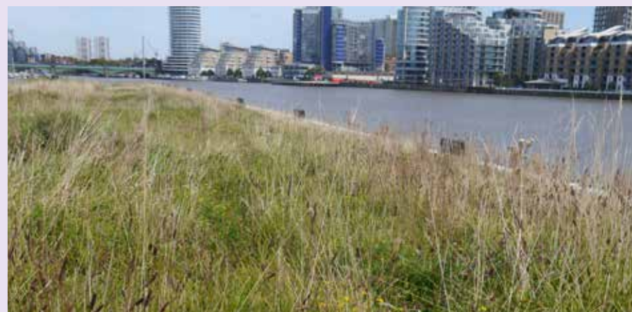
An extensive biodiverse roof provides habitat for invertebrates, some often rare, to feed and breed
