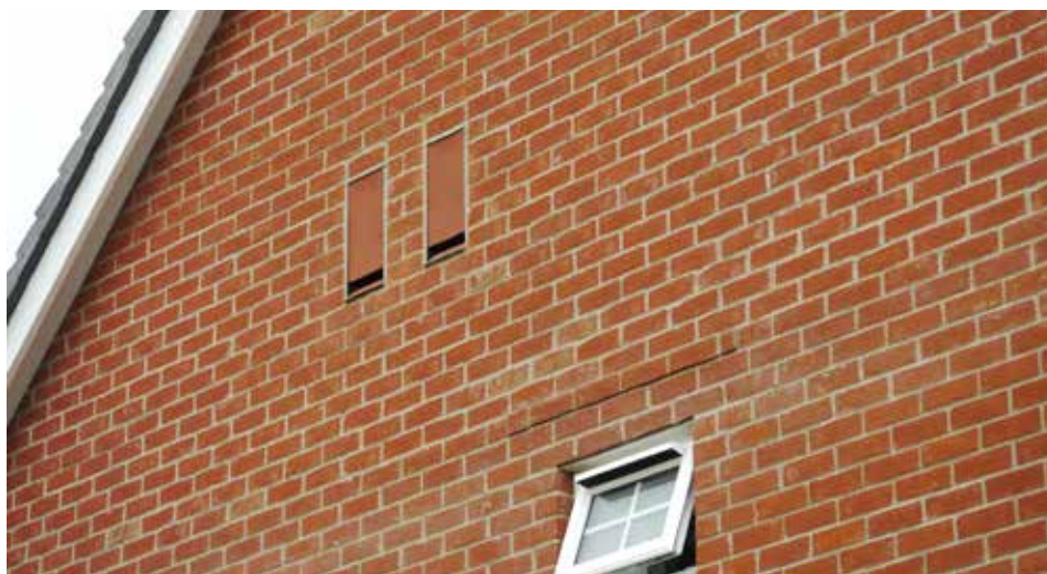
Figure 22 Bat bricks located above the habitation
