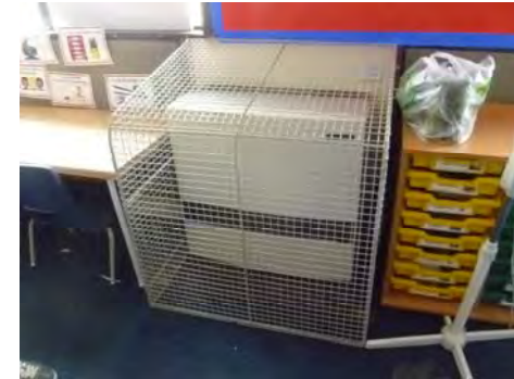
Nursery building heating
