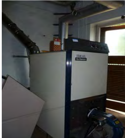
Boiler room Number two
