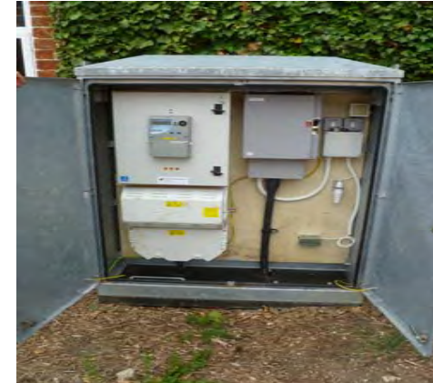
Main electrical supply Number two
